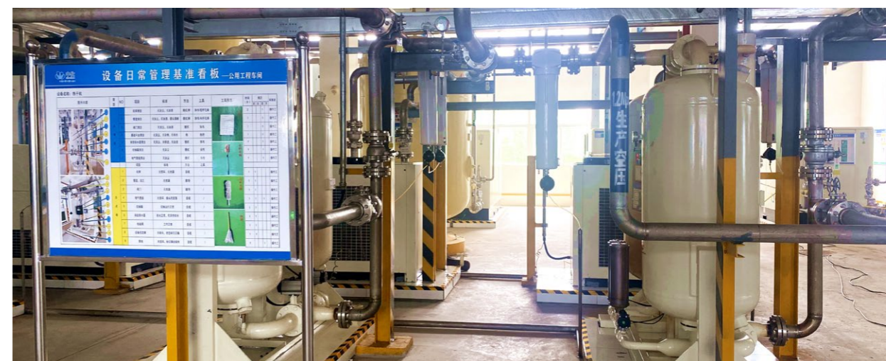
Air-pressure system post retrofitting as part of the joint energy-saving project with public works of Sinochem High Performance Fiber
