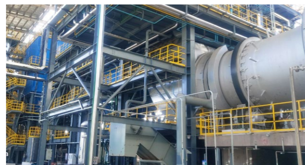
Yangnong Ruitai hazardous waste incineration
